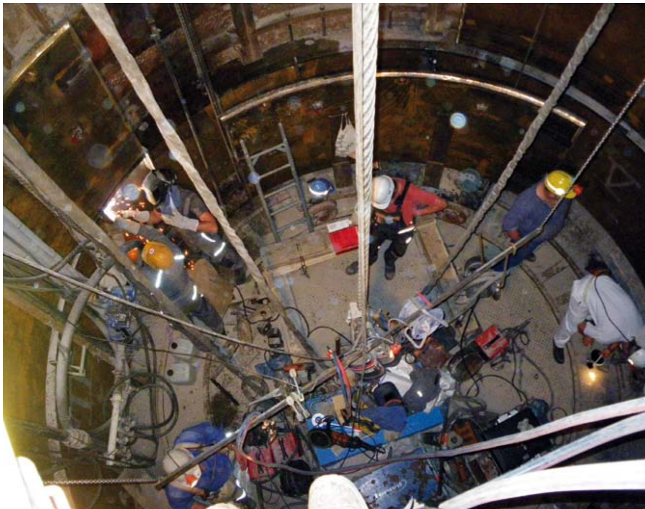
Abb. 9: Arbeits- und Brandschutzbühne in 294 m Teufe / Workers and fire safety stage in a depth of 294 m
